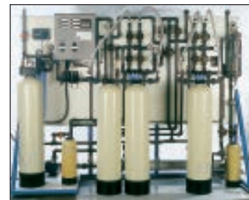
Open frame mounted deionizer/ultrafilter system-biomedical application
